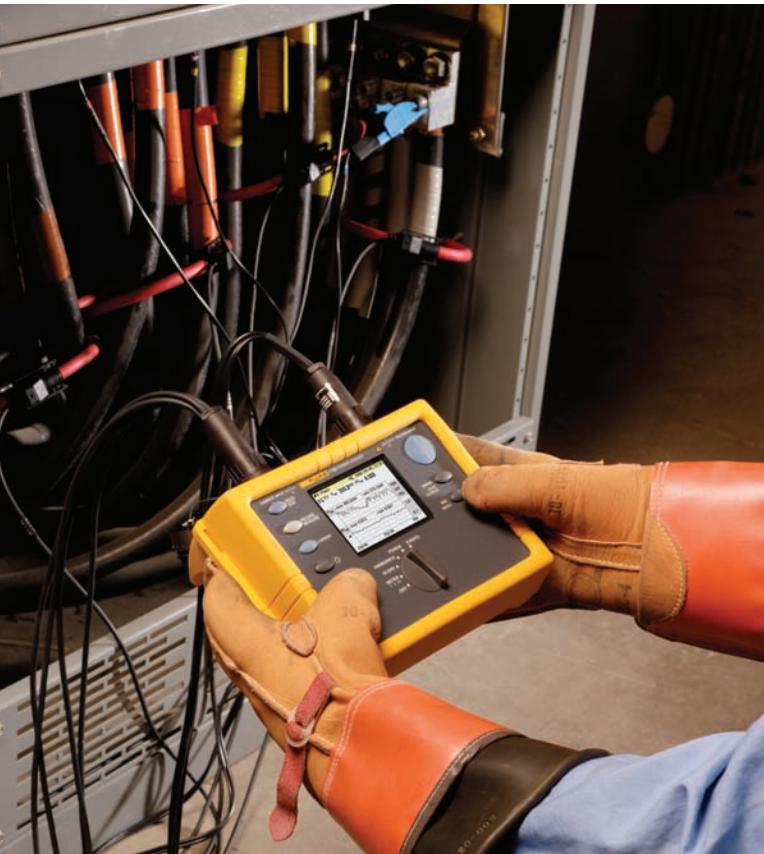
Setting up a Fluke 1735 Power Logger at the service entrance for a 30-day load study.
